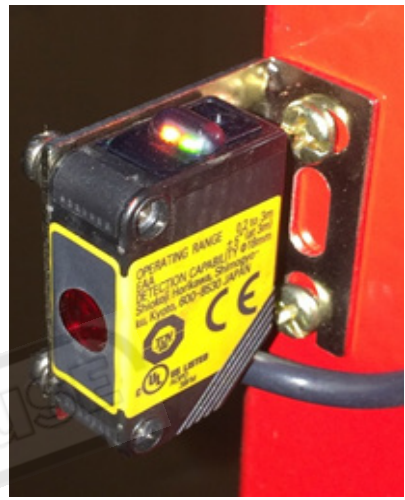
Has Power & aligned ok
